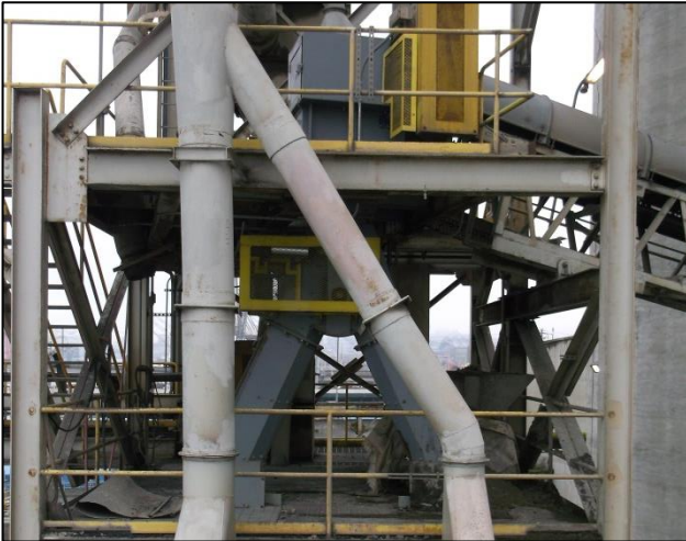
Figure 14. Ash Grove Cement Company, Seattle Plant, Proposed Design installed at TT6
